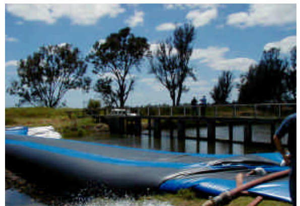
Water Corporations inflatable weir... a first for WA, being tested on the Capel River. It will be used to manage the flows next year during the weir replacement.
