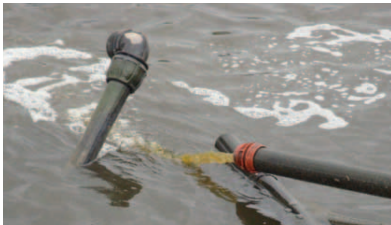
Clear effluent entering irrigation dam.
