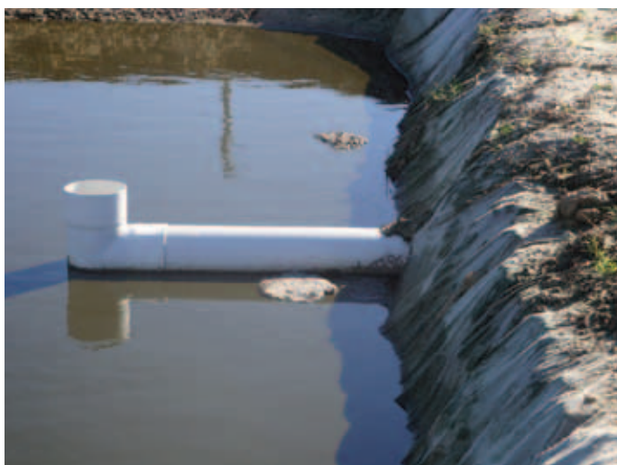
The "T" Piece on the effluent pond
