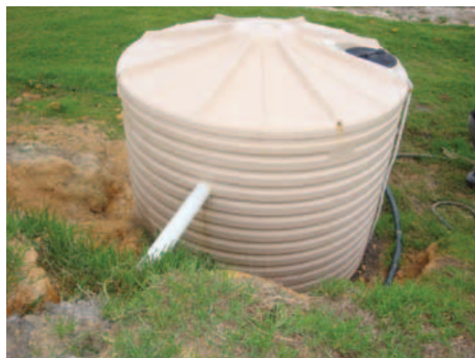
The effluent holding tank. T Piece pipe seen entering tank (90mm PVC stormwater pipe)
