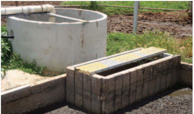
A retrofitted trafficable sump. Note vertically positioned boards. The new sump can be seen behind the trap in the background.
